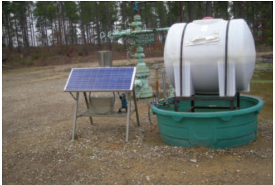
Figure 2. The iChem Solar Chemical Injection System installed at a well-head site.
